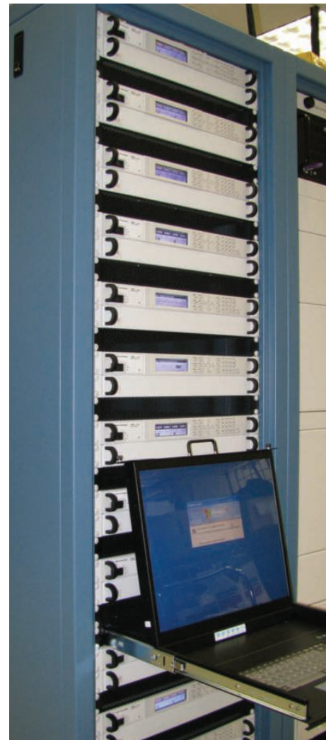
Figure 6: Custom turnkey system
